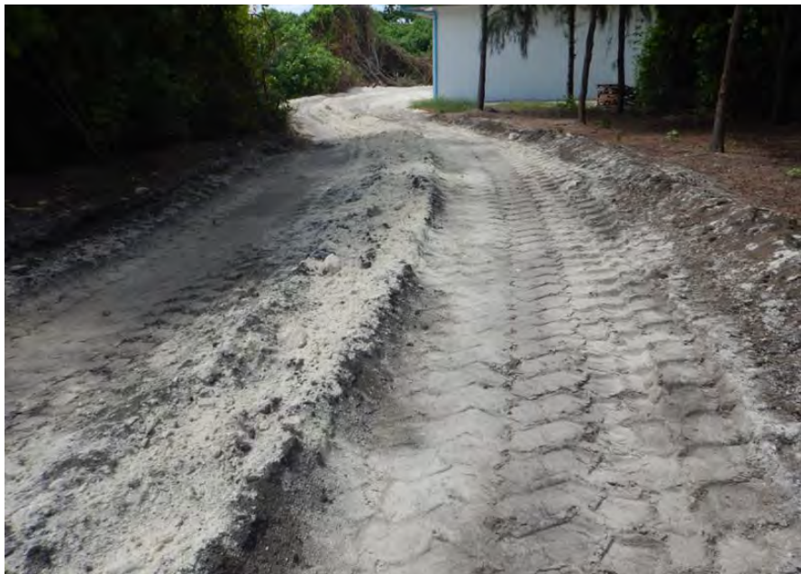
Figure 18: Impact on roads from heavy vehicle transport in an island in Maldives (Adapted from Saleem 2018)
