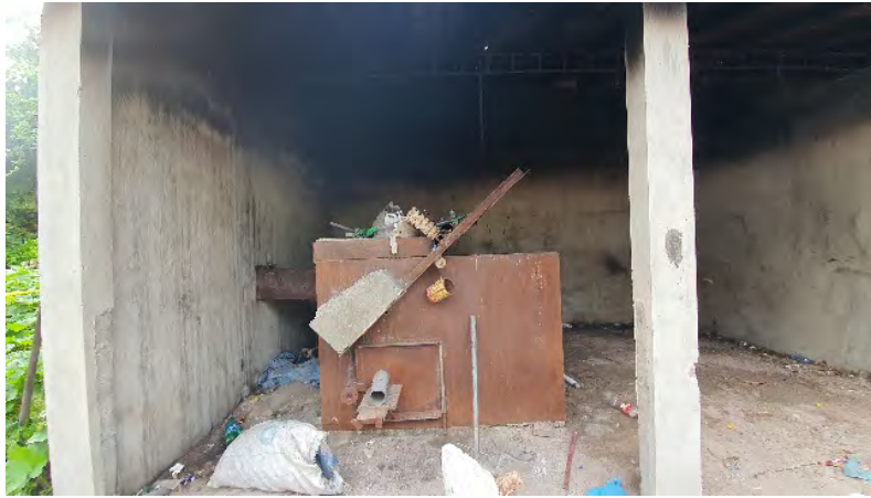
Figure 7. IWRMC Site; collection bays (top), Equipment and materials required for operation of IWRMC (centre) and Incinerator (bottom)
