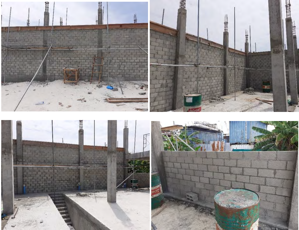
Workshop (These unapproved blocks have been removed now)
