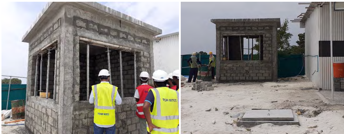
Guard Room (These unapproved blocks have been removed now)
