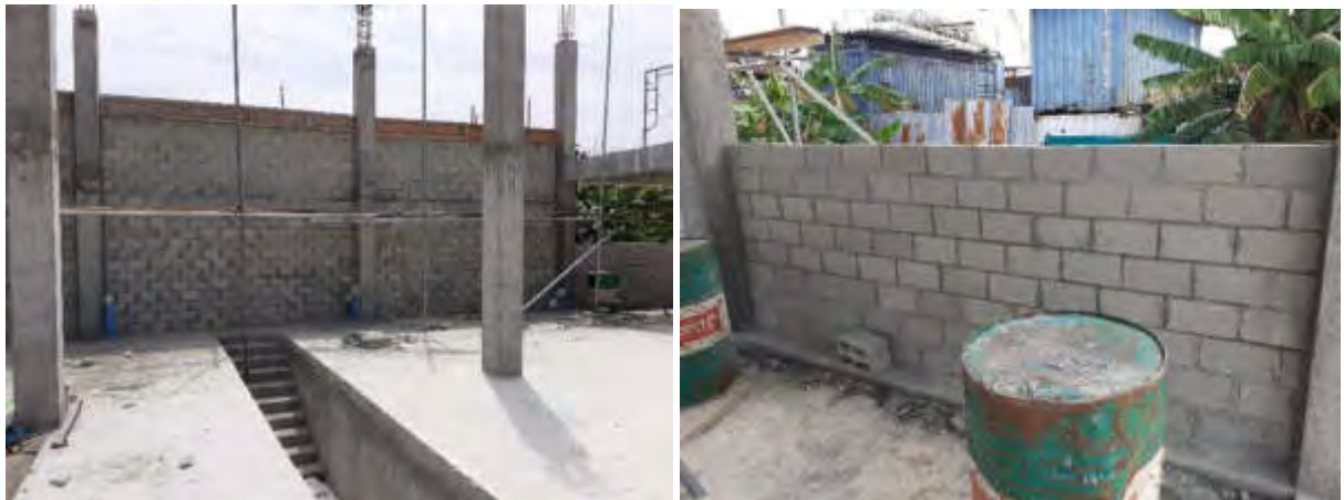
Workshop (These unapproved blocks have been removed now)
