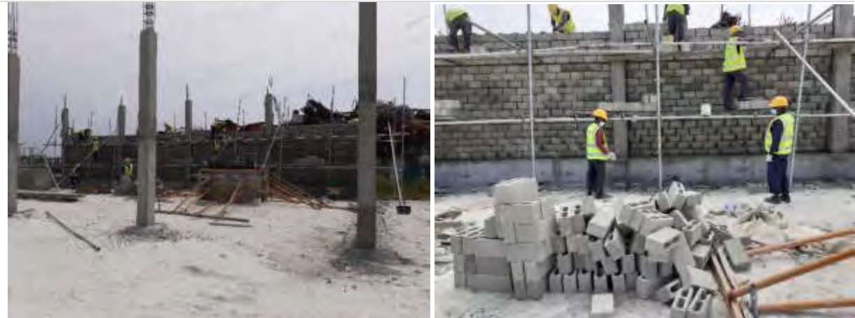
Parking shed (These unapproved blocks have been removed now)
