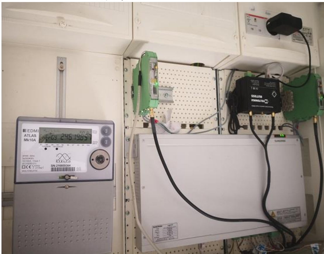
(Metering Device and Data Logger)
