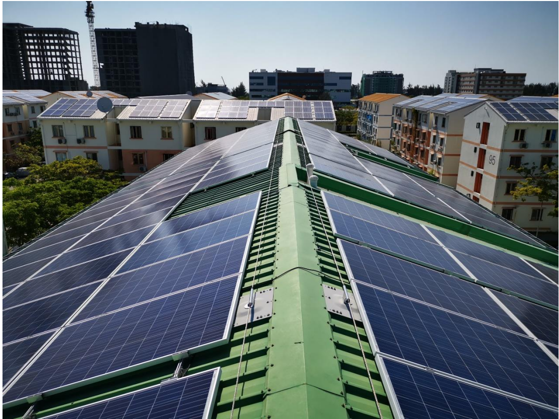
(PV Arrays on Roof)
