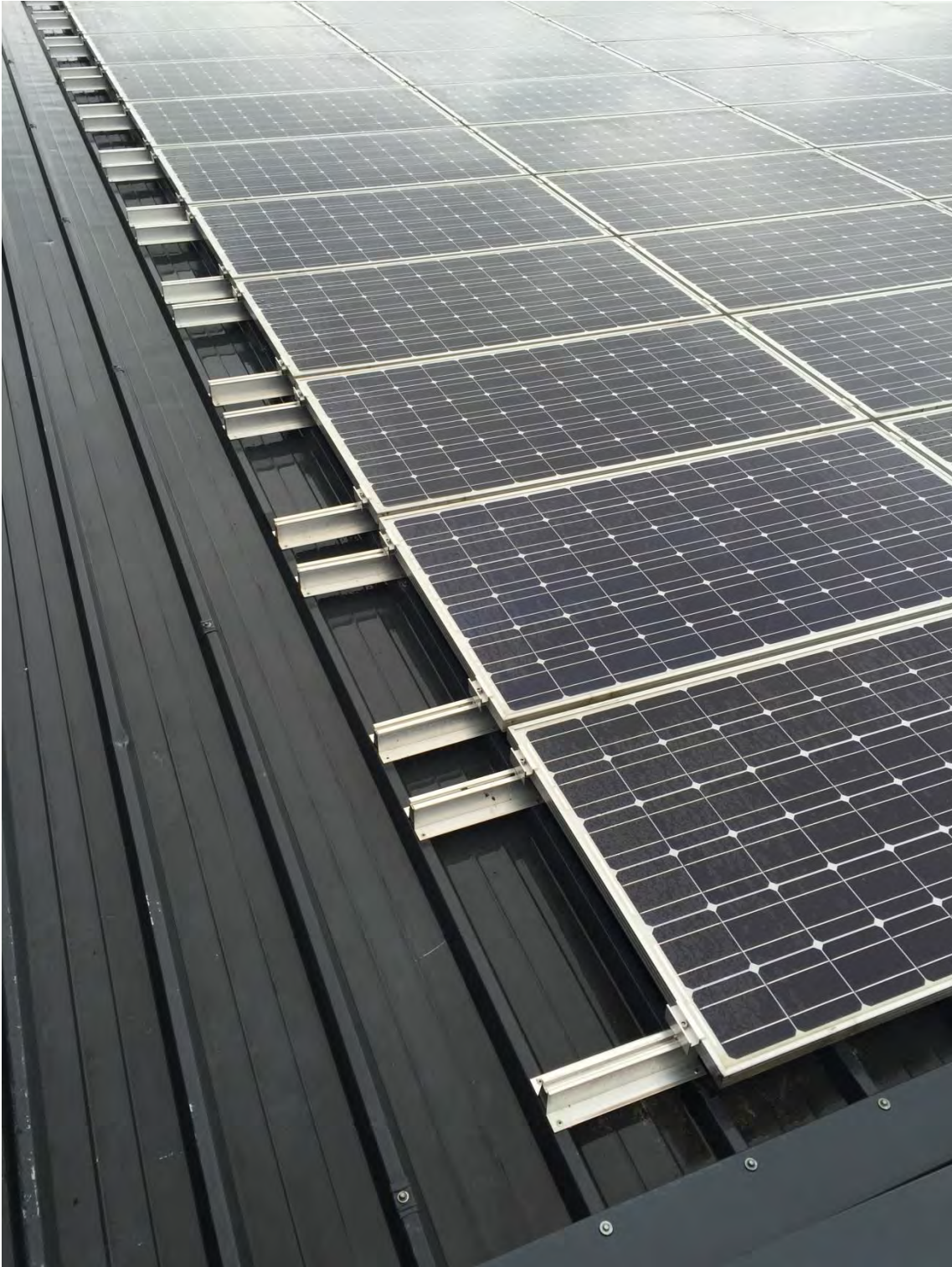
Figure 8: Substructure crossbar with PV modules
