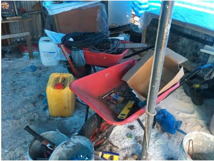
Figure 6 Wheelbarrows used by a contractor to transfer material from harbour to site
