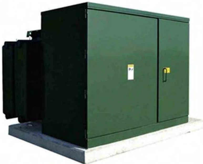
FIGURE 10 TRANSFORMER ON CONCRETE SLAB
