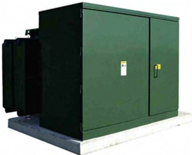
Figure 8: A transformer on concrete slab
