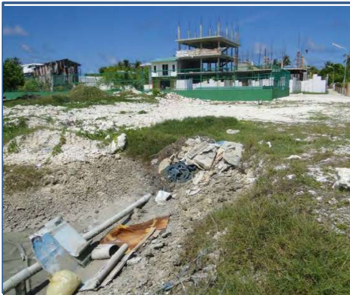
Existing out fall has to be rehabilitated by constructing flap gate cum culvert
