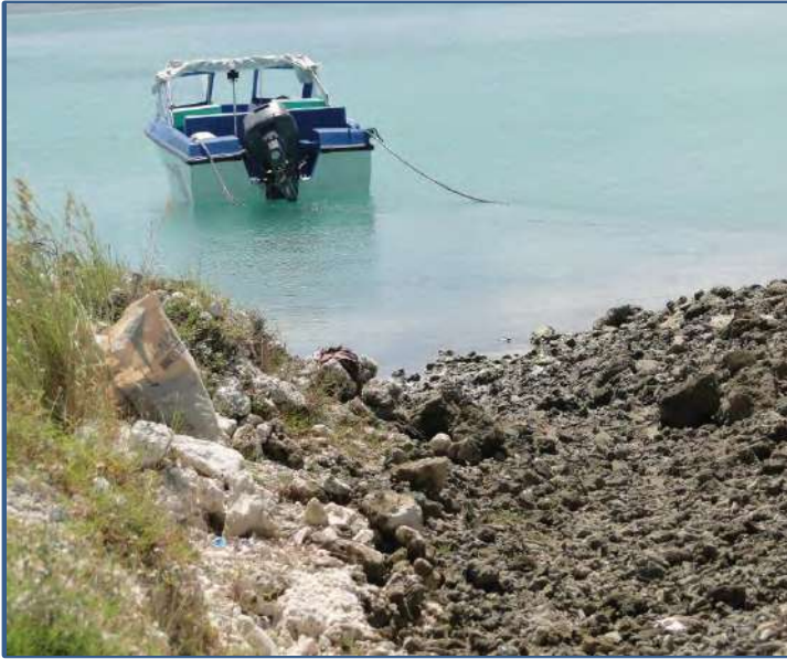
Existing out fall to be rehabilitated after constructing culvert cum flap gate
