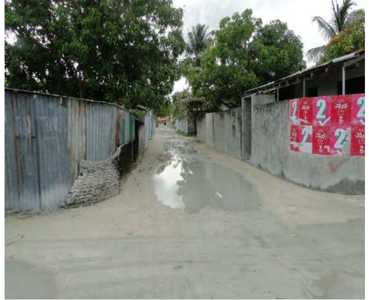
Link road to be filled to match the slope towards as main drainage path along the main road
