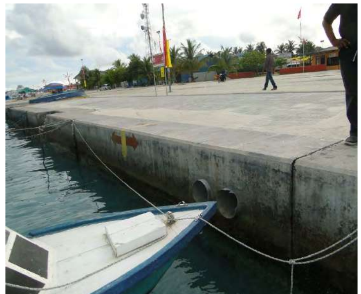
Flap gate has to be design to prevent salt water intrusion into inland area
