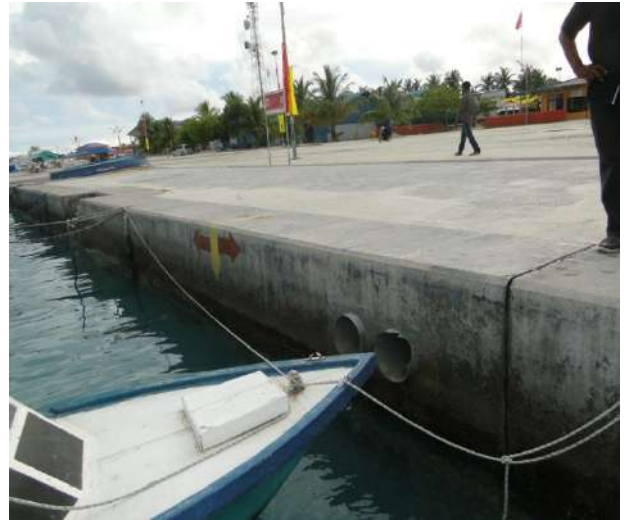
Existing emergency outlet location 02 Zone D
