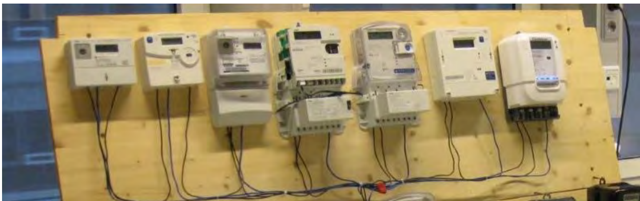
Figure 31: Submeters for different end uses in a building
