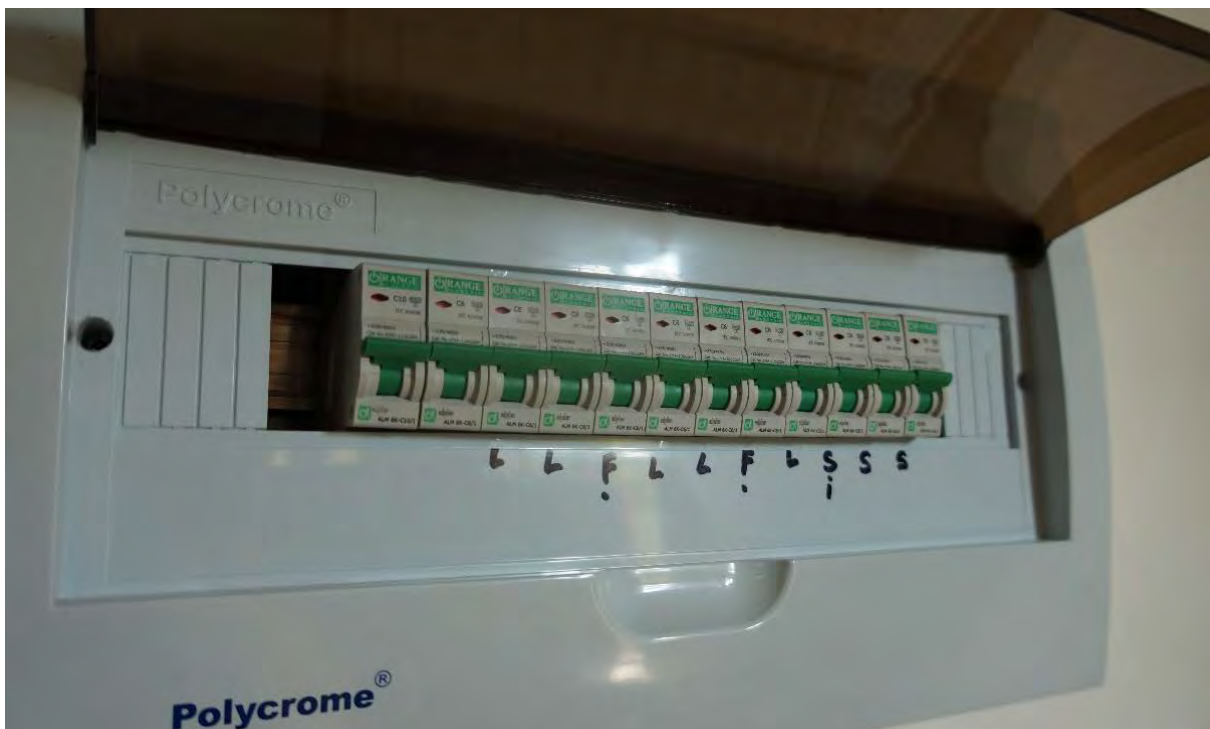
Figure 3-3: Typical Internal Electrical Distribution Centre Showing Multiple Uses Downstream
