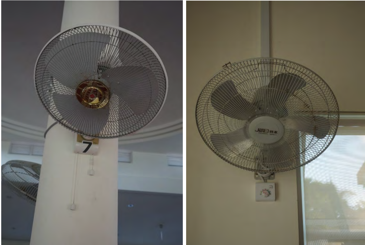
Figure 1-5: Existing wall fans in Masjid-ul Sidheeq
