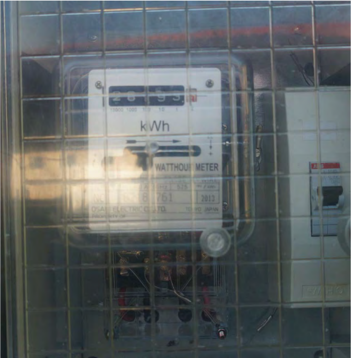
Figure 1-13: Existing single phase power board at Masjid-ul Sidheeq
