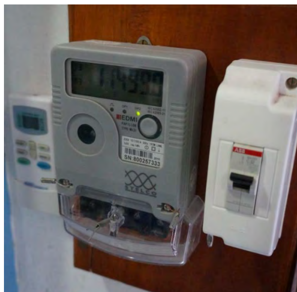
Figure 3-1: Internal Check Meter
