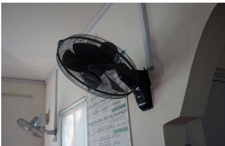
Figure 1-16: Existing wall fans in Masjid-ul Sidheeq
