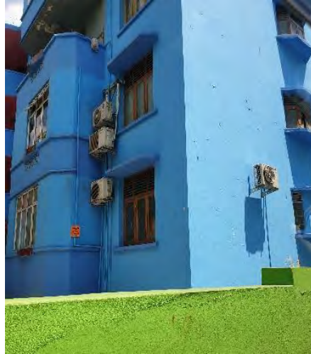
Figure 21: Image showing outdoor units of split air conditioning systems
