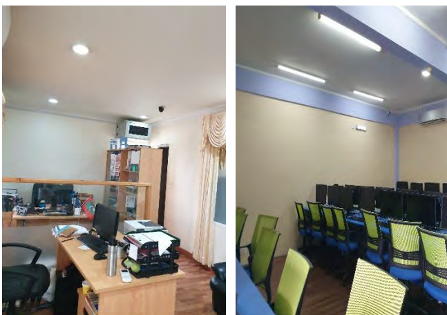
Figure 157– Images showing LED lighting installed in the office area and computer lab
