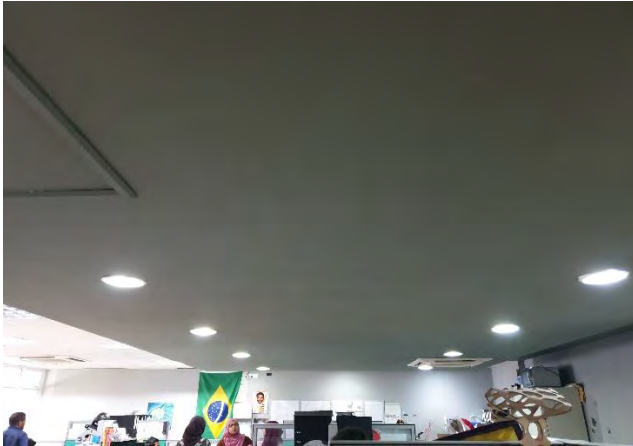
Figure 130– Image showing LED lighting installed in the workspace
