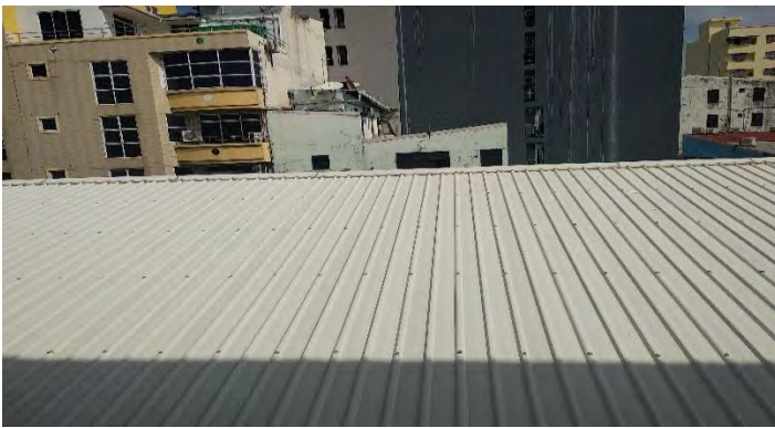
Figure 92– Adjacent building white Tin roof reflects high amount of glare inside the building
