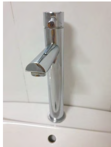
Figure 226– Image showing faucet in toilets
