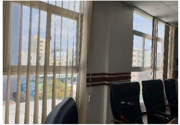
Figure 91 – Image showing usage of Internal blinds in Conference rooms
