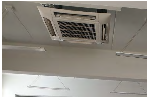
Figure 96– Image showing cassette air conditioners
