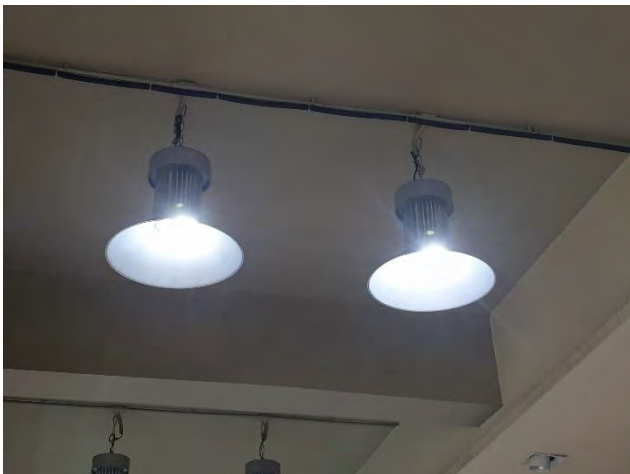
Figure 167– Image showing LED lighting installed in the supermarket
