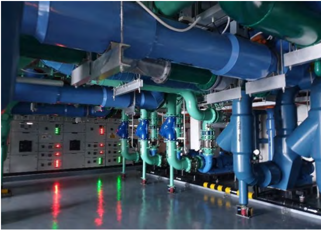
Figure 120– Image showing Chiller Plant Room
