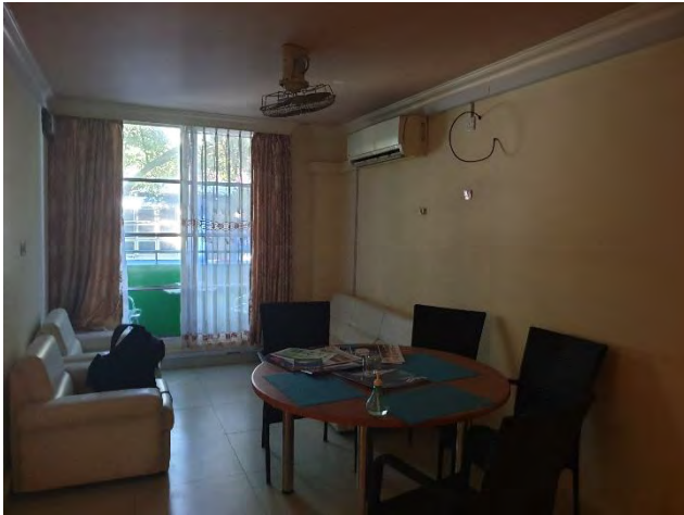
Figure 223– Image showing wall mounted split ACs in reception area
