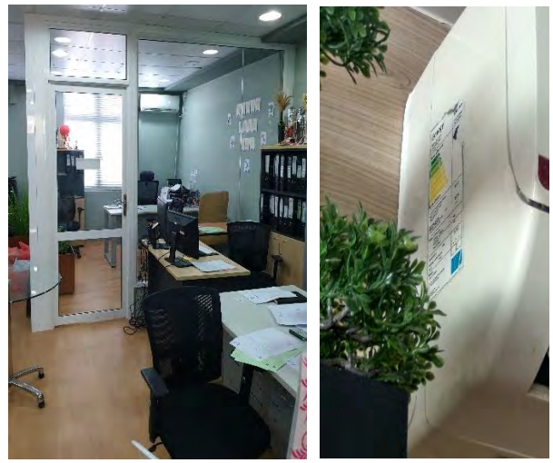
Figure 133– Images showing wall mounted AC in cabins & its specification
