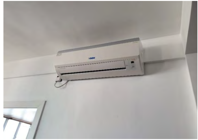
Figure 195– Images showing wall mounted ACs installed in the apartment
