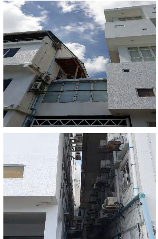
Figure 87 – Image showing North and South sides of ME building with adjoining buildings on both sides
