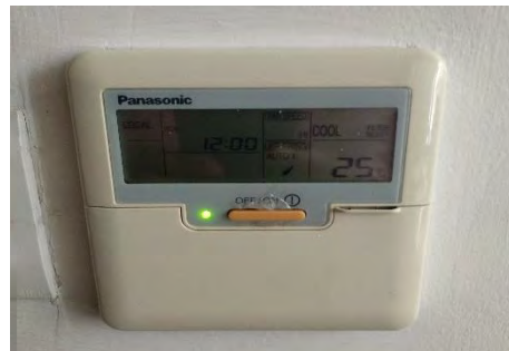
Figure 98– Image showing set-points of 25 deg C set in the workspaces. Awareness on high setpoint is issued by Energy Department.
