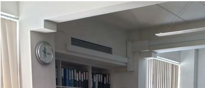
Figure 97– Image showing non-operational air ducts in the building due to mold and fungus problems in chilled water.
