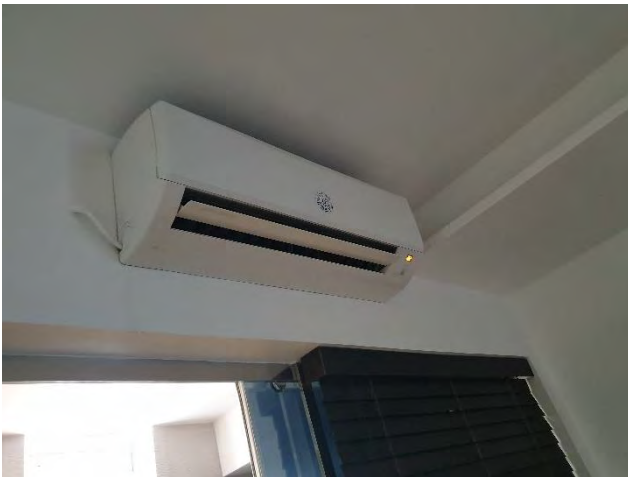
Figure 213– Image showing wall mounted split ACs in guest rooms
