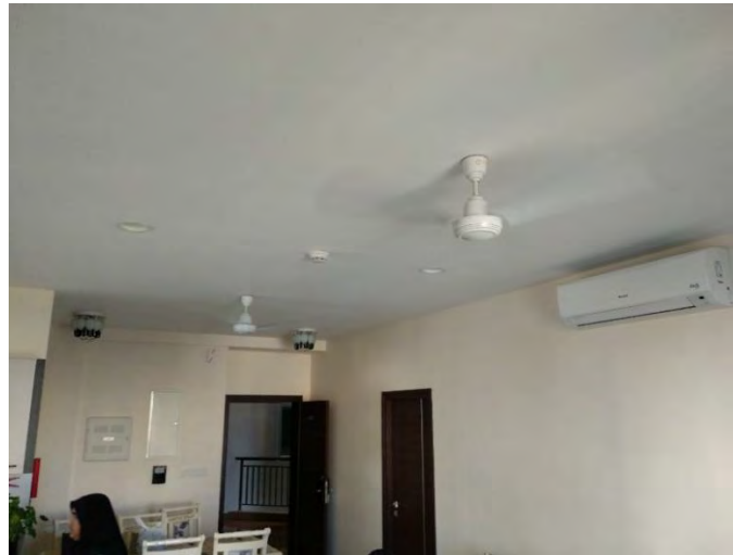
Figure 204– Image showing fan and wall mounted AC installed in the apartment
