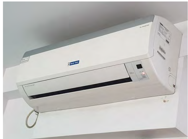
Figure 201– Image showing wall mounted AC installed in the apartment
