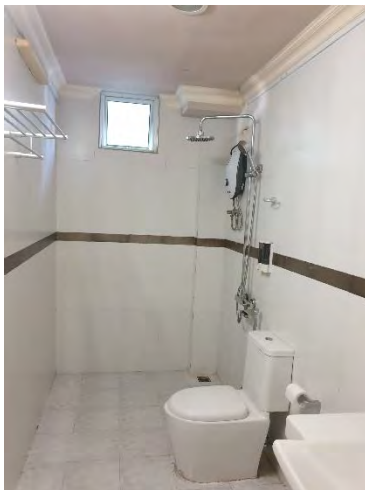
Figure 225– Image showing Dual flush fixtures
