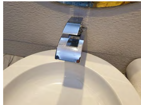
Figure 216– Image showing faucet in toilets
