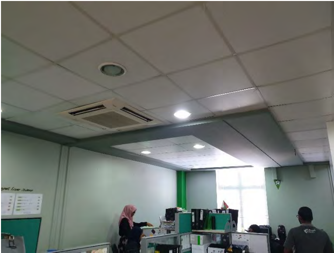
Figure 132– Image showing wall mounted AC in workspace
