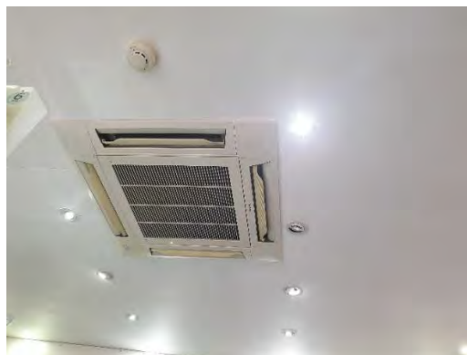
Figure 175– Image showing ceiling mounted AC in one of the shop
