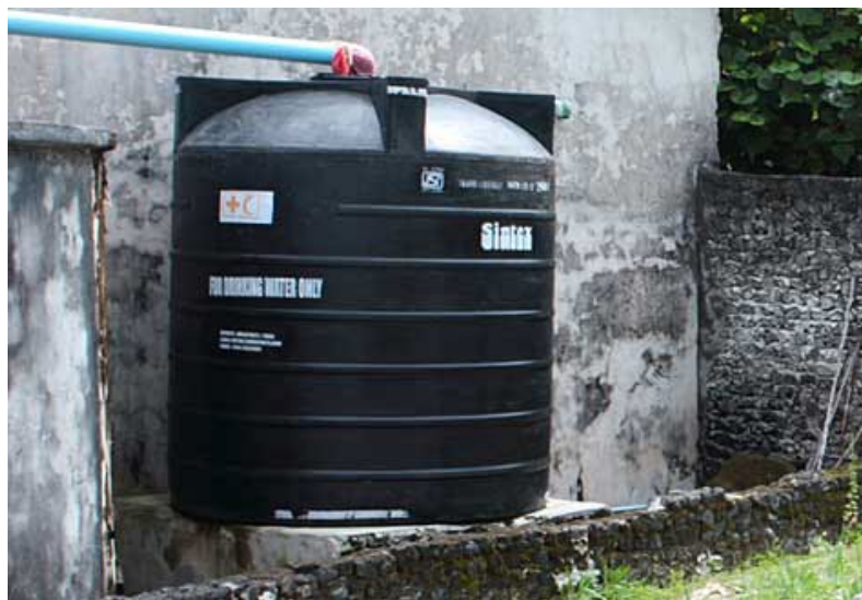
Figure 2.10: PVC pipes and a PE tank are connected to the roof to collect rainwater in a rainwater harvesting system installed on an island. (Source: www.bluepeacemaldives.org/blog/2009/03 )
