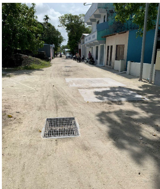
Figure 2.11: A catch pit of the stormwater drainage system installed on an unpaved sandy road of S.Feydhoo island. These systems can be clogged with waste and may carry other pollutants on road surfaces with them – (Source: Authors)
