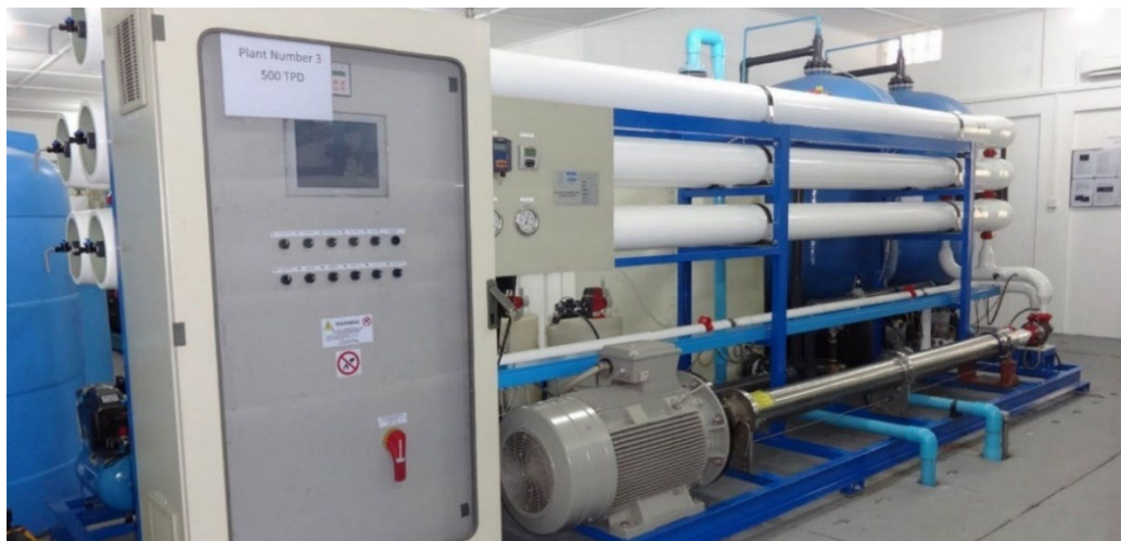
Figure 3.1: A desalination plant established on an island. (Source: kuredu.com)
