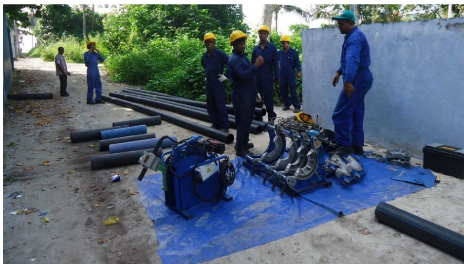
Figure 3.8: An ongoing operation to join HDPE pipes together by butt fusion welding. (Source: mwsc.com.mv)
