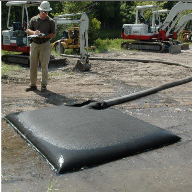
Figure 4.7: A settlement unit used for separating sediments from dewatering. Source: h-dewatering.ca (top). Dewatering bag is a solution that can be used to release dewatering output to the land (in case of less saline water) (bottom) source: https://spillcontainment.com/
