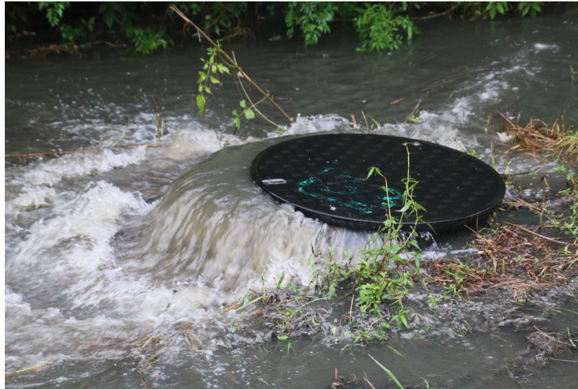
Figure 1.27. Sewage overflow from a sewer manhole – (Source: https://www.apr.org/post/alabama-probes-fish-kill-after-sewage-spilled-near-creek )
