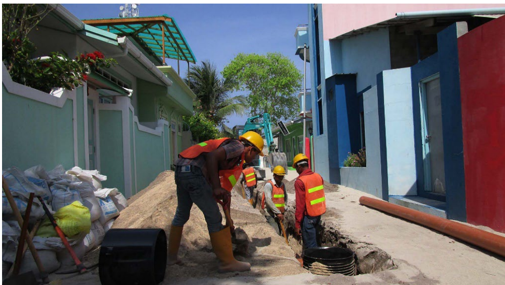
Figure 1.14: A conventional gravity sewer pipeline being constructed on an island in the Maldives – (Source: mwsc.com.mv)
