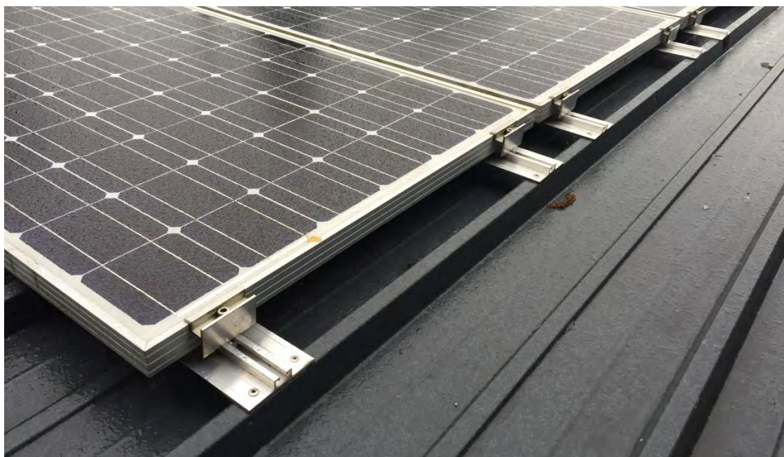
Figure 7: Example substructure crossbar with mounting clamp (end fitting) and PV modules
