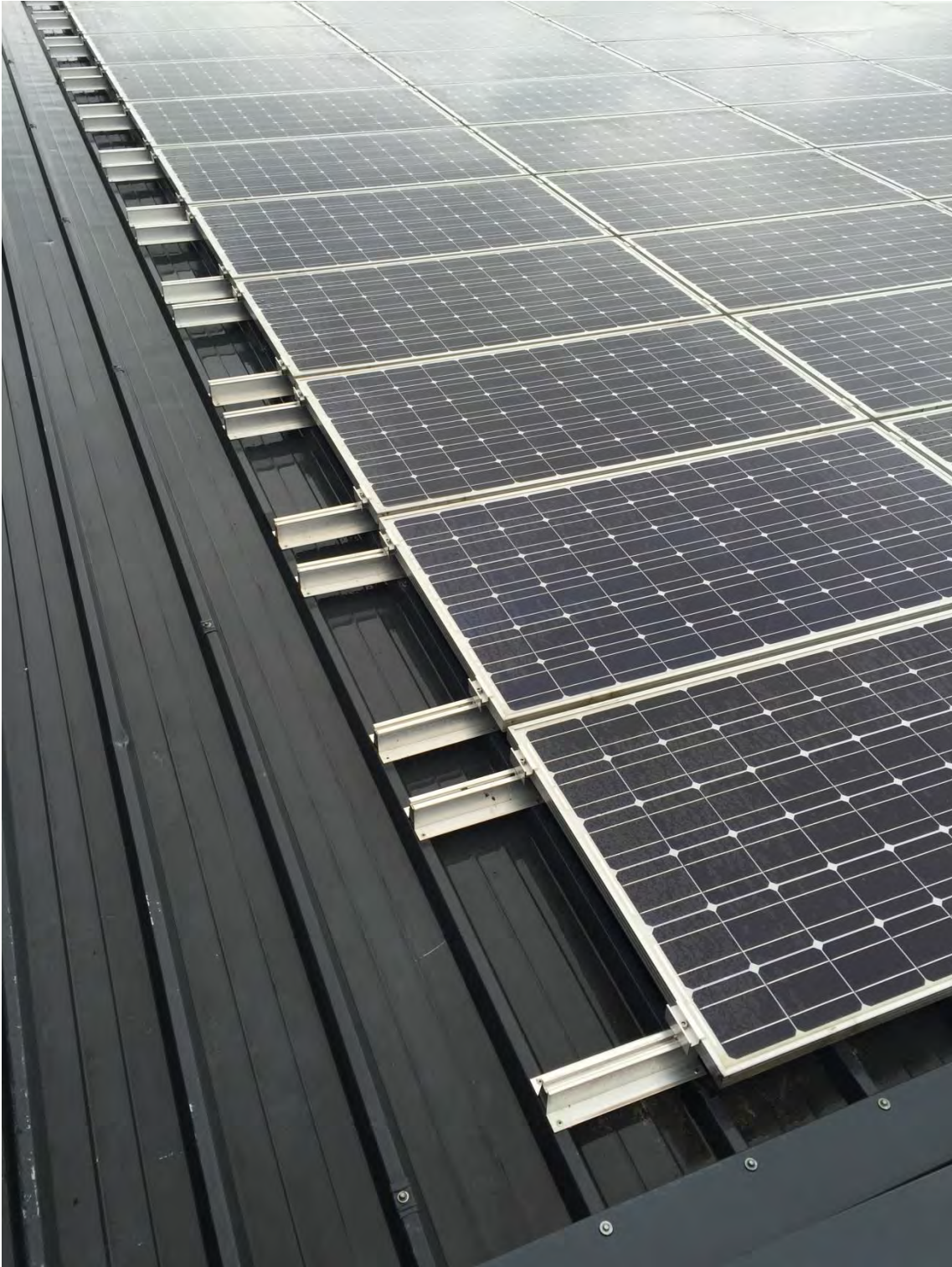
Figure 8: Substructure crossbar with PV modules
