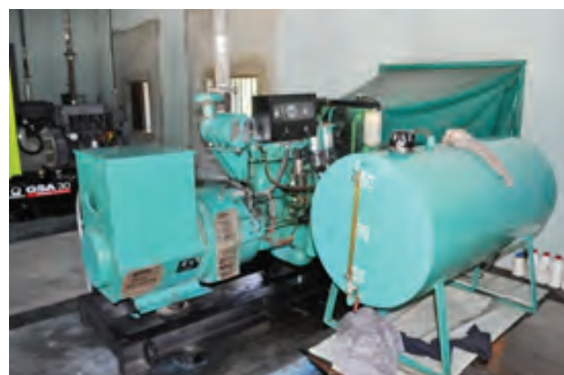
A diesel generator installed at a powerhouse
