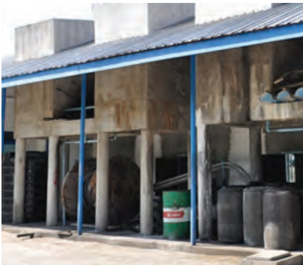
Fuel storage at the back of the power house at an island
