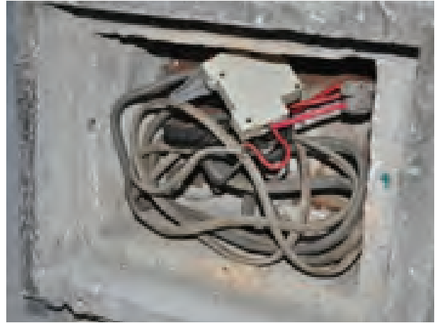
Distribution box at an island
