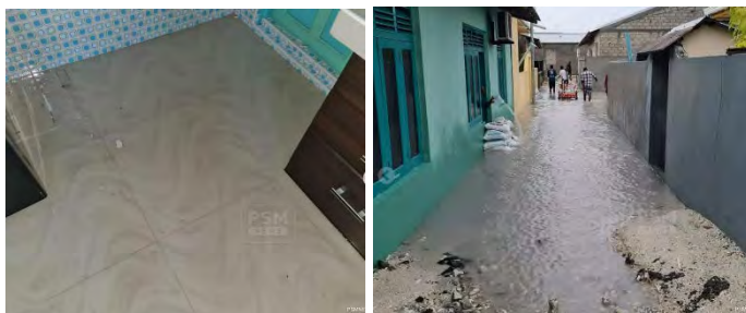
Figure 19 Damages caused by squally showers in Ha. Dhidhdhoo on 14th May 22. Source: PSM
