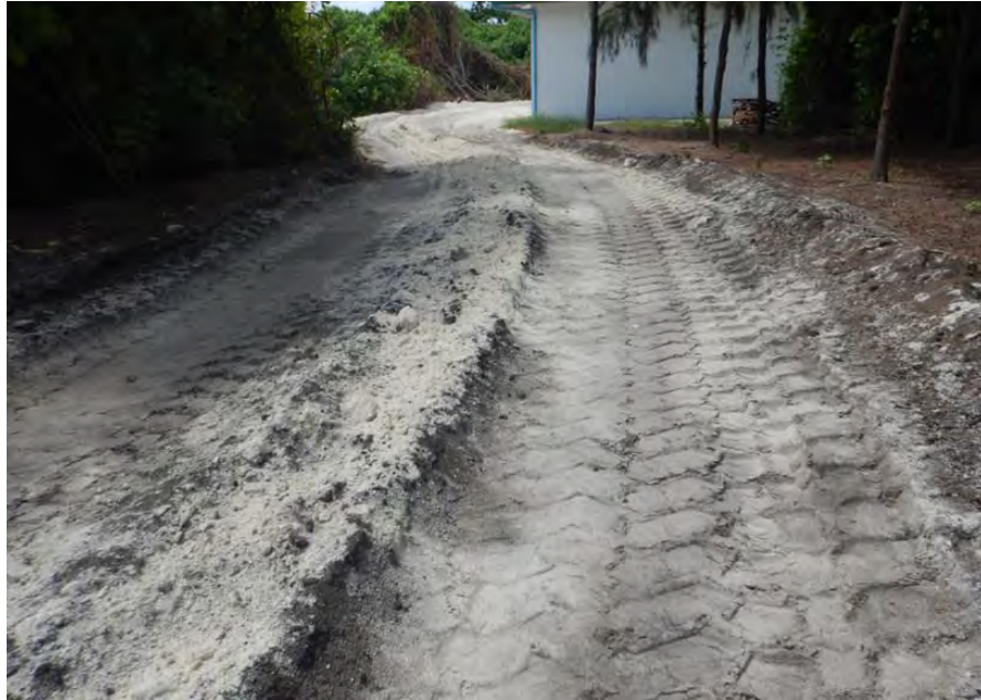
Figure 17 Impact on roads from heavy vehicle transport in an island in Maldives
