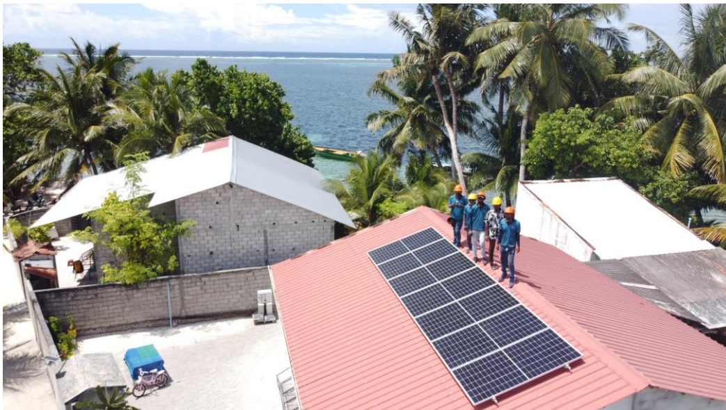
Solar photovoltaic systems installed on a rooftop.
