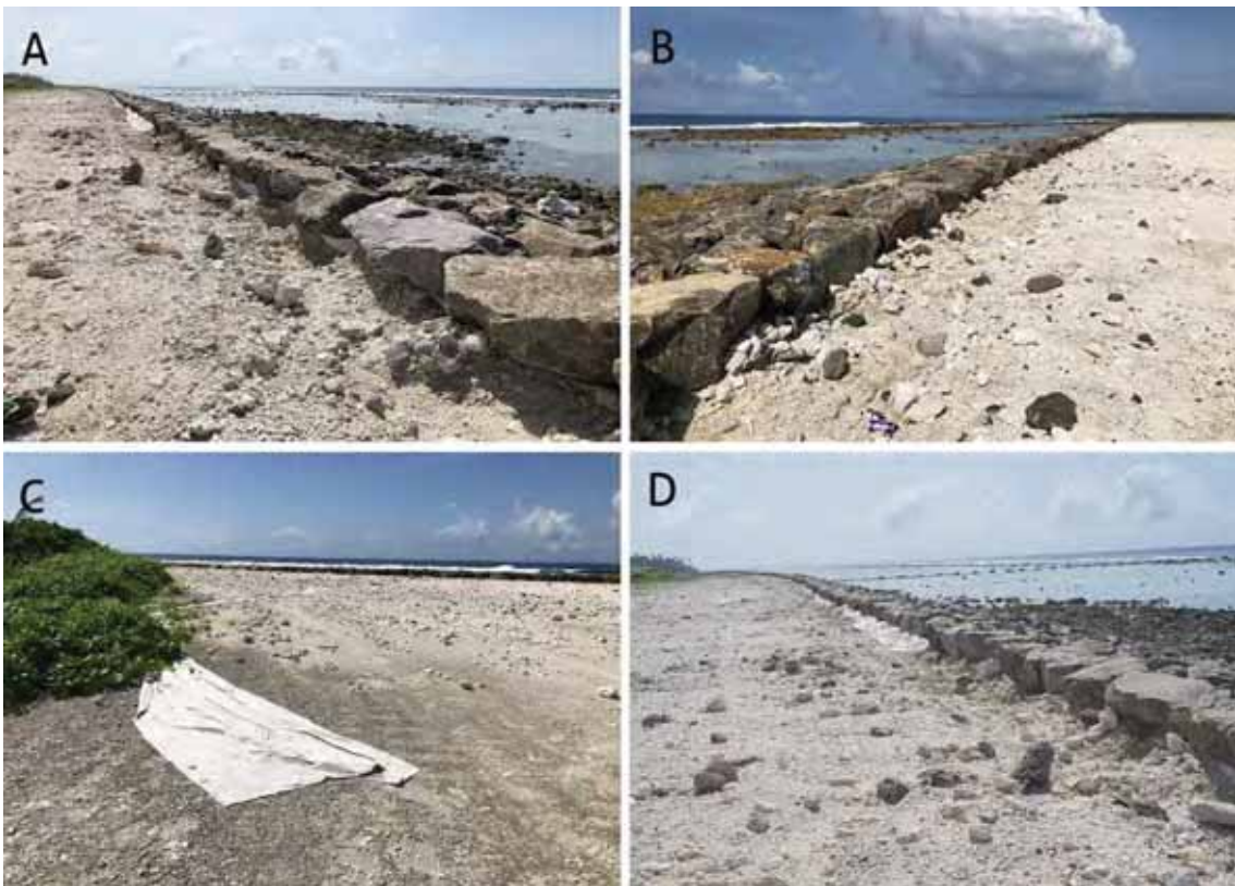
Figure 13: (A) to (D) Damage caused to the revetment and geotextile in recent 'udha' incident
