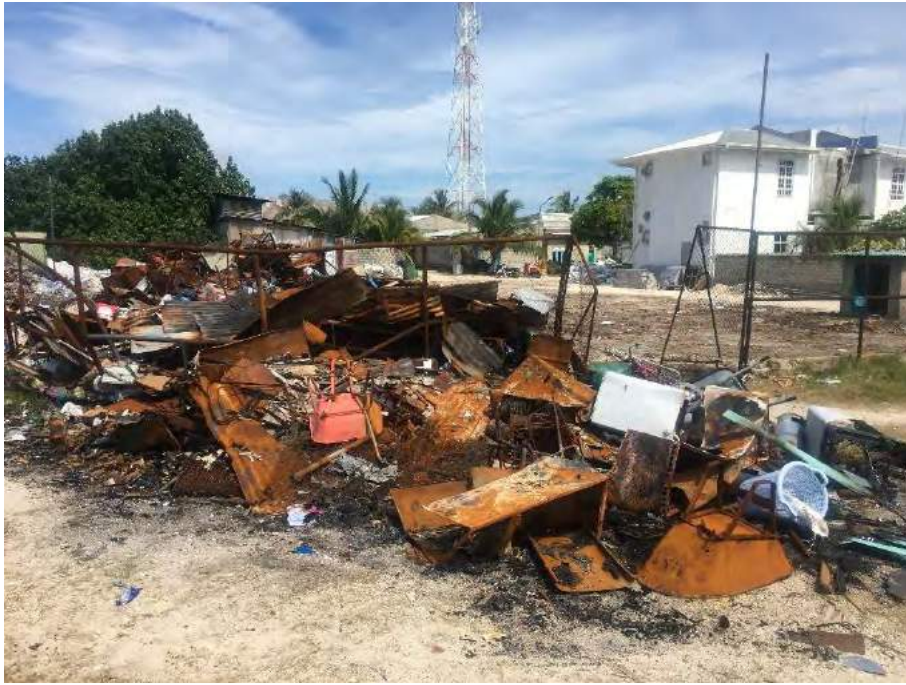
Figure 10 Metal waste pile at the site
